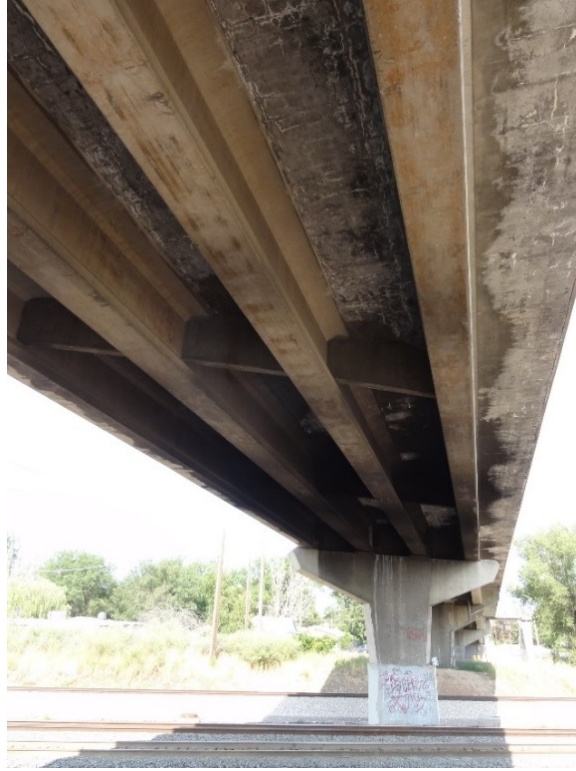
Figure 4-17: Significant efflorescence and cracking on the underside of the deck in case study #1.
